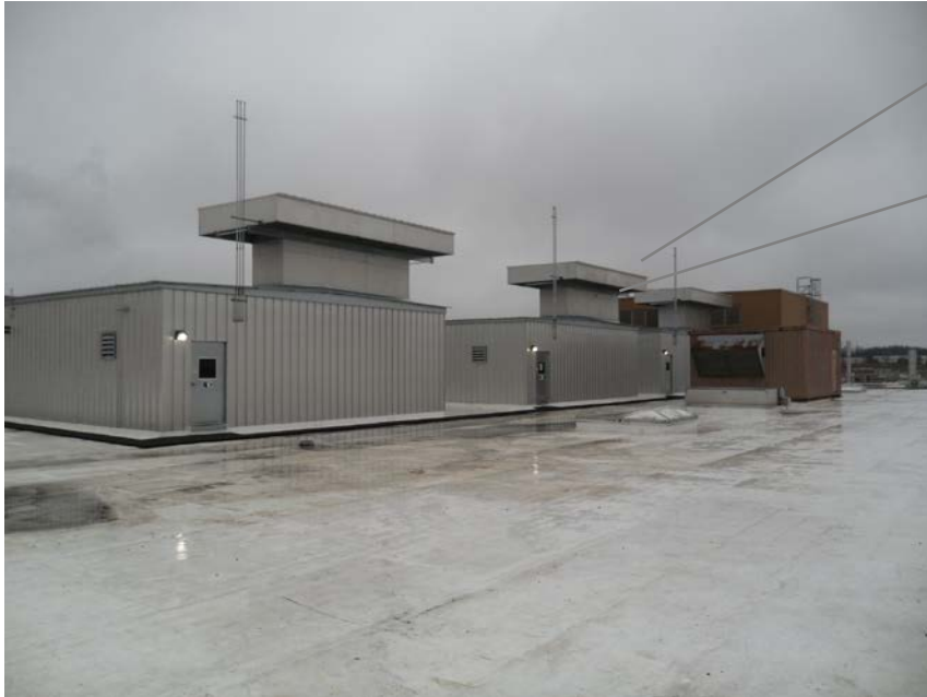
Air Supply Houses used for Makeup Air (On Roof of Paint Booth)
