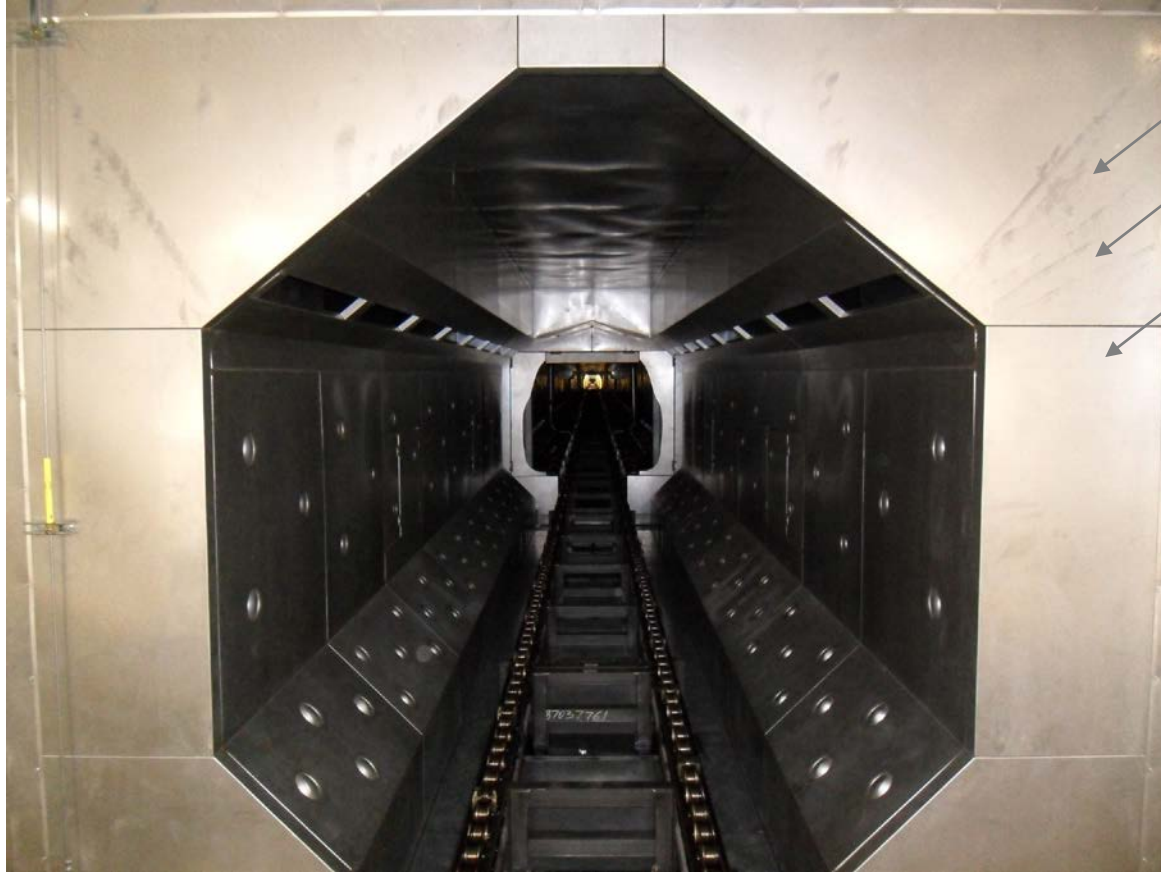
Paint Curing Oven
